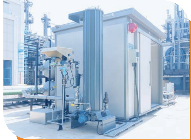
Extraction of hydrogen from town gas in Tai Po
