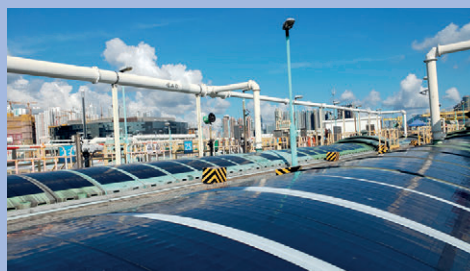
The thin-film solar PV system at Stonecutters STW
