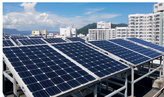
The solar energy generation system installed by the Housing Authority at Shui Chuen O Estate
