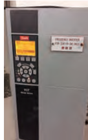
VSD installed in HVAC system
