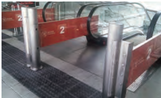
Service-on-demand escalators with passenger sensing post
