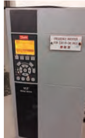
VSD installed in HVAC system
