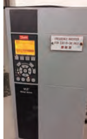
VSD installed in HVAC system
