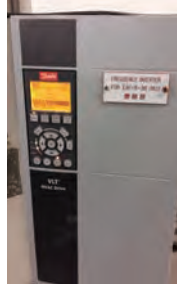
VSD installed in HVAC system
