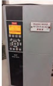
VSD installed in HVAC system
