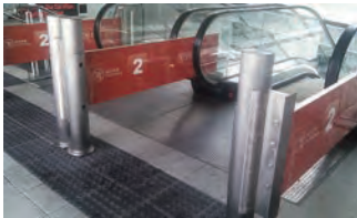
Service-on-demand escalators with passenger sensing post
