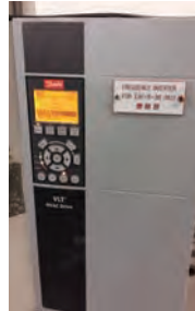
VSD installed in HVAC system
