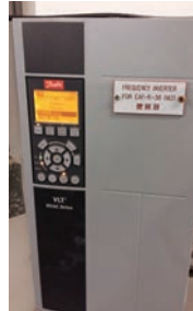
VSD installed in HVAC system
