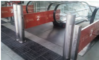
Service-on-demand escalators with passenger sensing post
