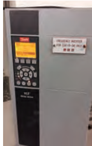
VSD installed in HVAC system
